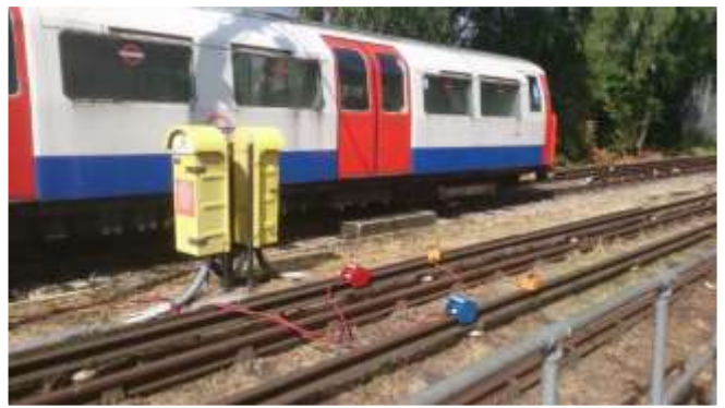
Earth Fault Test Boxes
