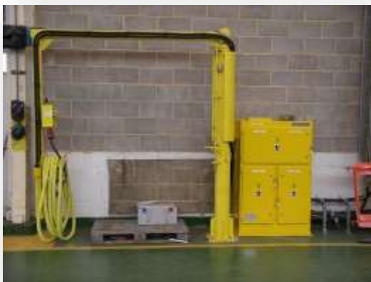
Parked Overhead Boom
