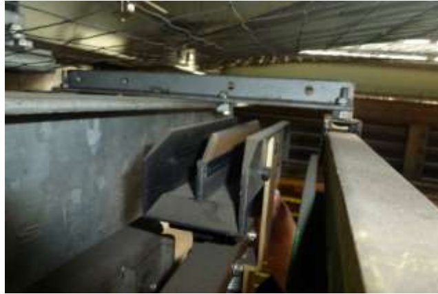
Contactor panels components after 10 years on load use in a London Underground Depot
